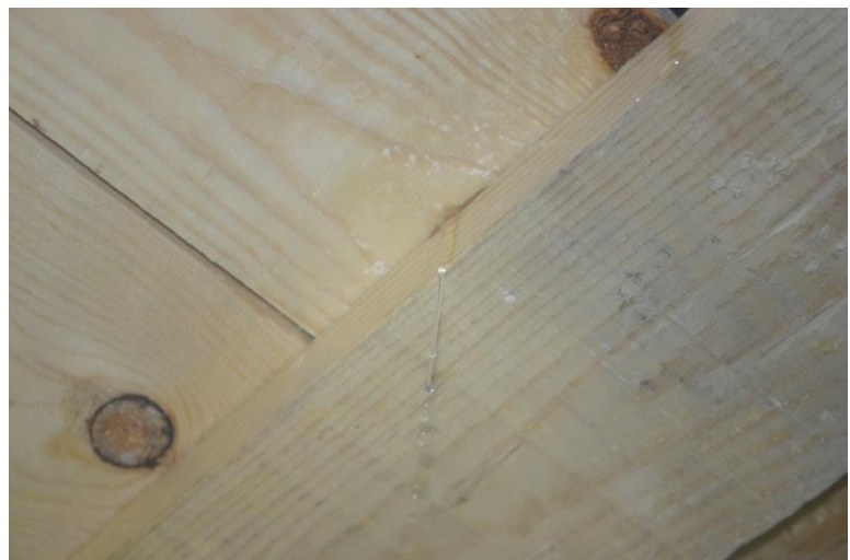
Photo 9 Leakage which occurs at wind-rain combination B (with extra wind and extra water) on test specimen 1 at a slope of 7,5°.
